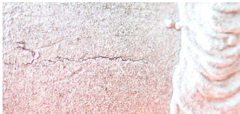
Figure 22: Potential Stress Corrosion Cracking on Feeder 3 Valves
