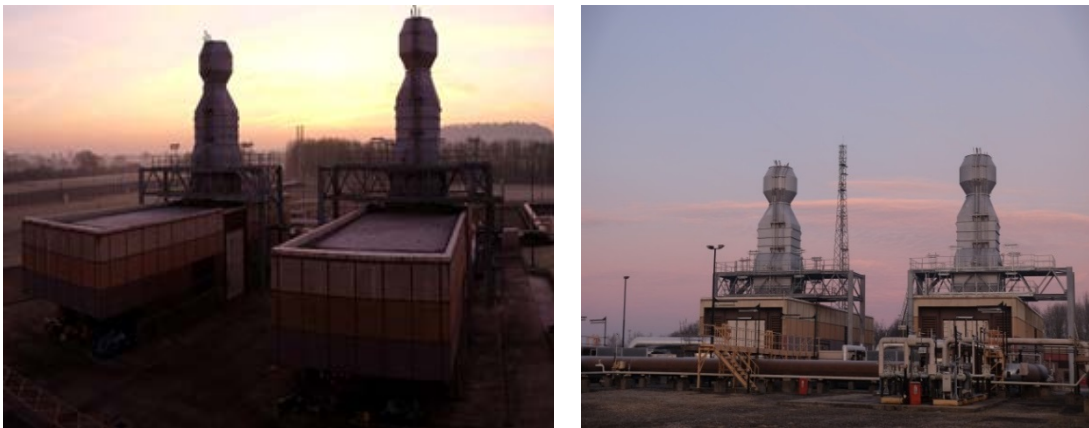
Figure 32: Exhaust stack and catalyst abatement system at Aylesbury compressor station
