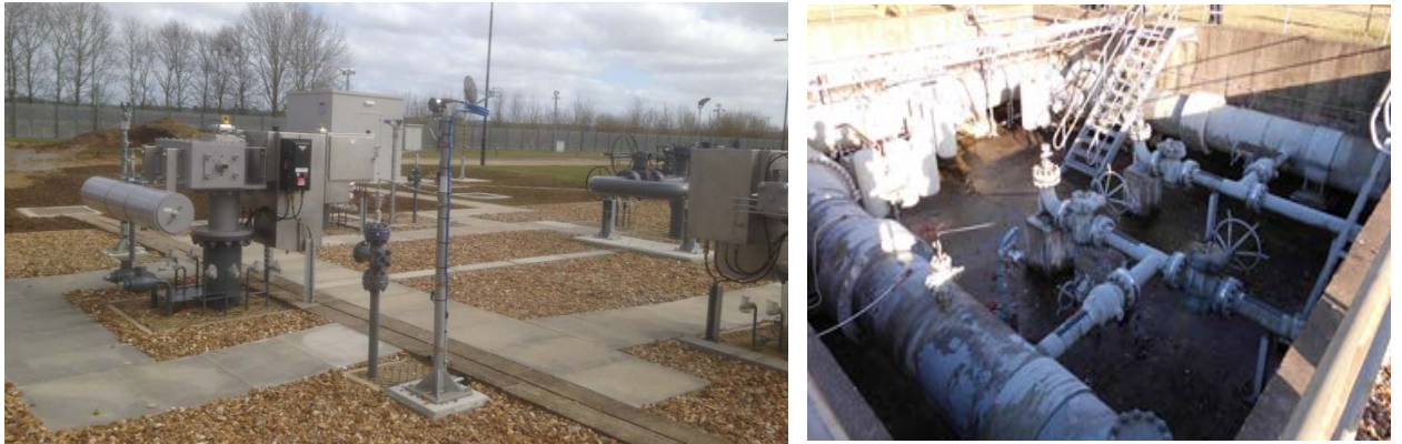
Figure 21: New Cambridge Tee (left); Previous Cambridge Tee Pit (right)
